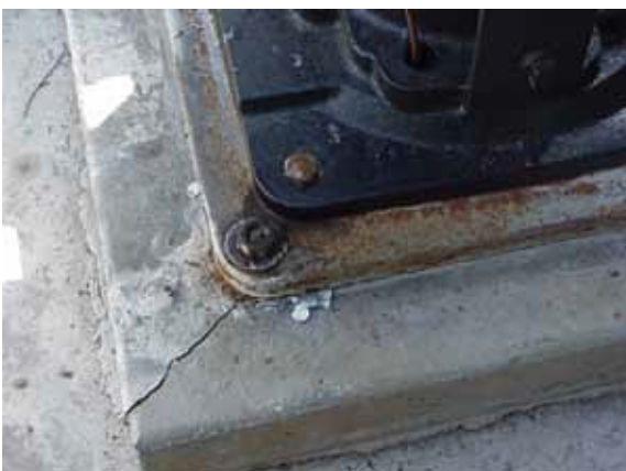
Figure 10. Vertical Turbine Pumps – Improper Installation
