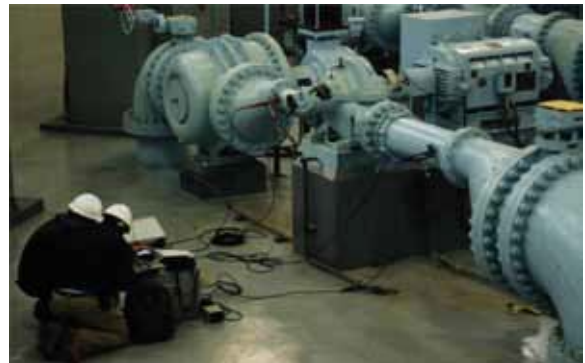
Figure 4. Elevated Pump Unit
