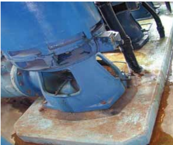
Figure 9. Vertical Turbine Pumps – Proper Installation
