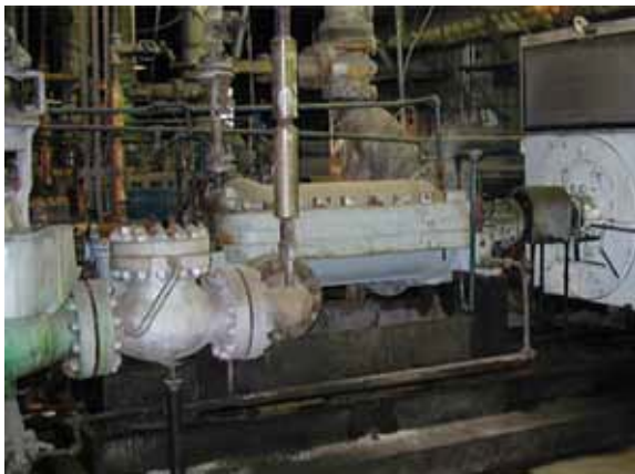
Figure 1. Boiler Feed Pump Unit
